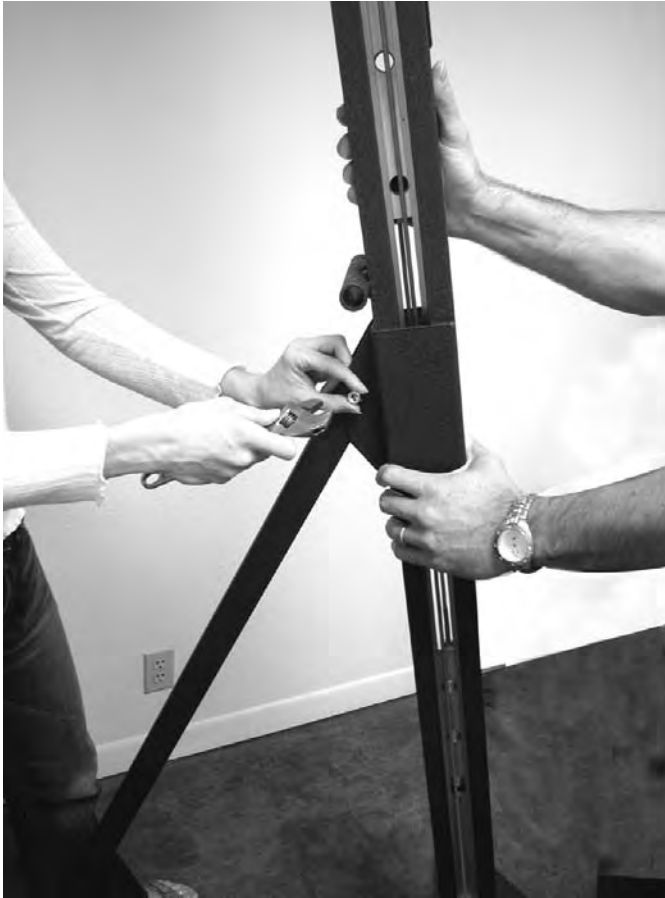
With another person holding at a slight angle, assemble the brace and tie to the post.
